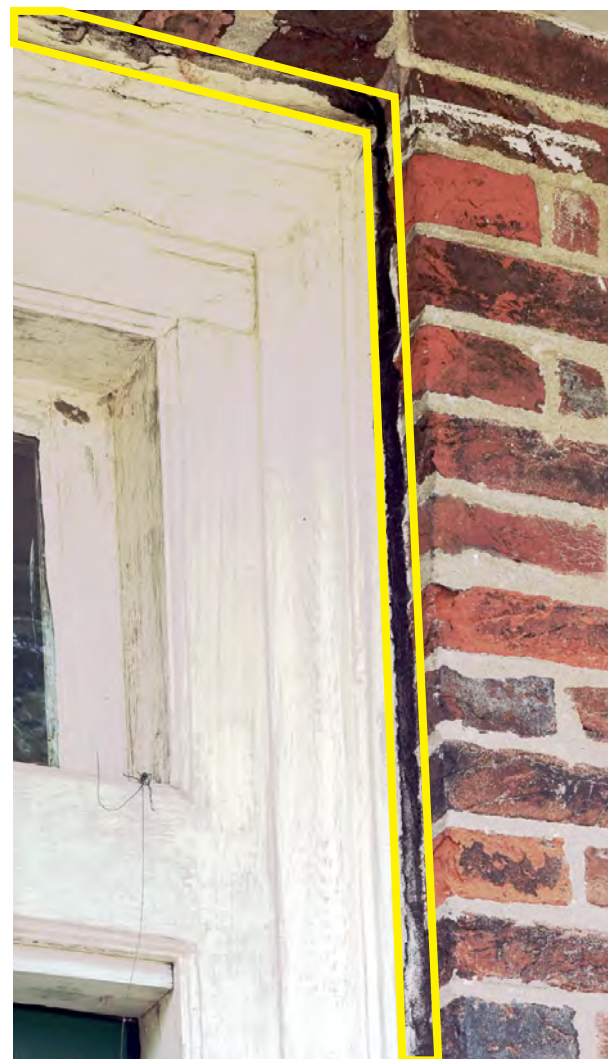
E CAULK & SEALANT REPLACEMENT EXAMPLE OF WHERE DETERIORATED OR INAPPROPRIATE CAULK NEEDS TO BE REMOVED, TYPICAL FOR ALL BUILDING AREAS. REPLACE WITH BACKER ROD WHERE NEEDED AND SEALANT OR CAULK PER SPECIFICATIONS.
