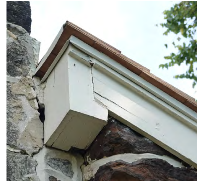
C WOOD REPAIRS AT ROOF REPAIR FASCIA & RETURN CORNICE MOLDINGS AT SHED ROOF. FILL HOLE IN MASONRY W/ BACKER ROD, TUCK POINT & CAULK BETWEEN WOOD & MASONRY
