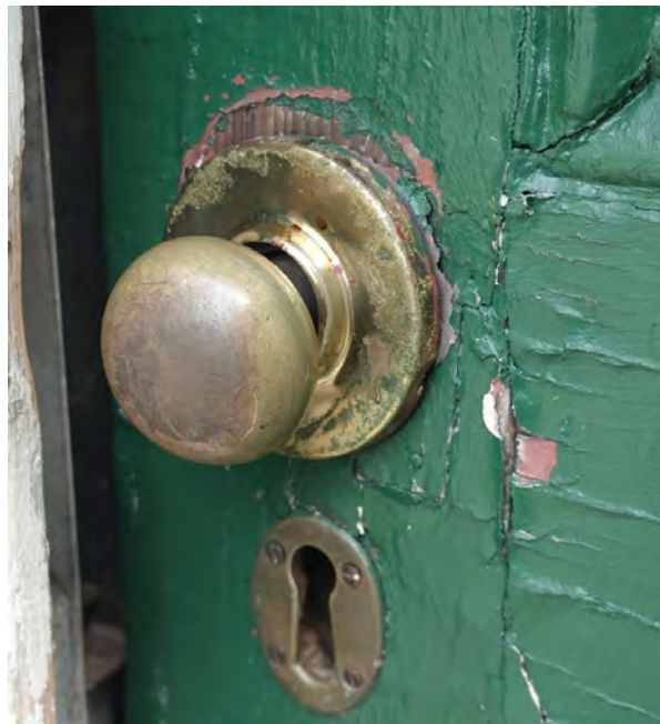
D EXTERIOR DOOR HARDWARE RESET DOOR HARDWARE AFTER REPAIRS TO DOOR, SECURE ESCUTCHEON.
