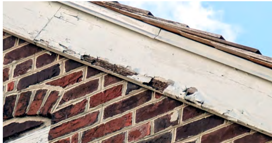
E WOOD REPAIR REPAIR GABLE END RAKE BOARD
