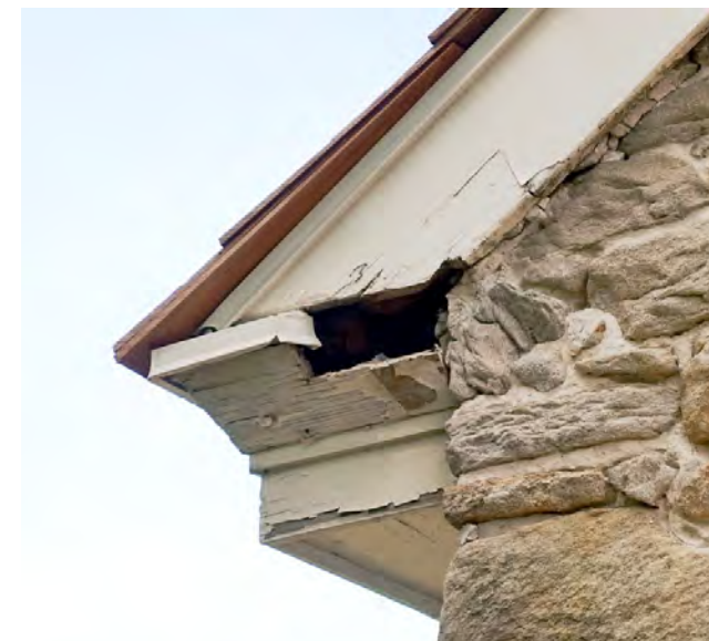
A WOOD REPAIRS @ CORNICE REPAIR CORNICE RETURN TO MATCH CONFIGURATION OF OPPOSITE (EAST) SIDE
