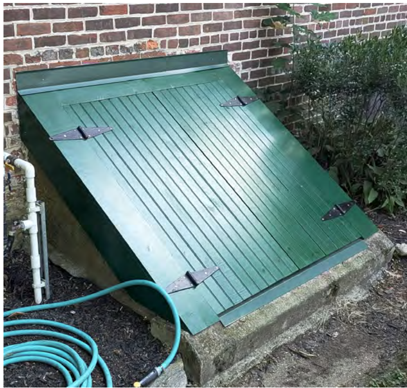
E WOOD REPAIRS - BULKHEAD DOOR INSTALL ASTRAGAL ON RECENTLY INSTALLED BULKHEAD DOORS
