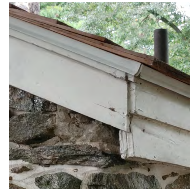
D WOOD REPAIRS @ ROOF REPAIR FASCIA. INSTALL MISSING TRIM TO MATCH RETURN ON OPPOSITE (EAST) CORNER
