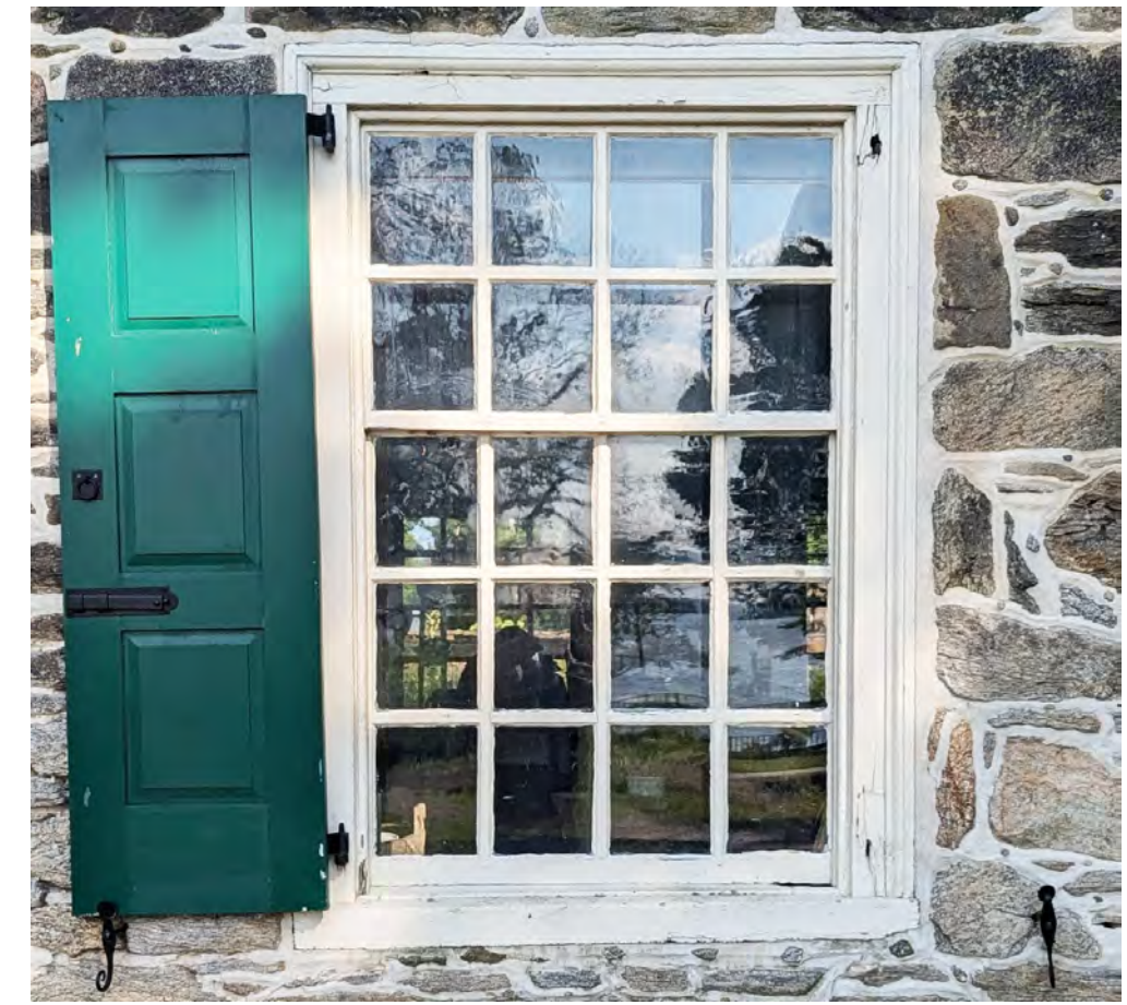
A WINDOW w/ MISSING SHUTTER & PINTLES
