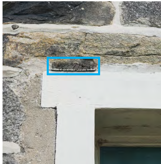
E EXTERIOR ABOVE DOOR REMOVE EMBEDDED PIECE OF WOOD ABOVE DOOR HEAD. FILL w/ BACKER ROD, MORTAR & CAULK JOINT @ WOOD DOOR FRAME
