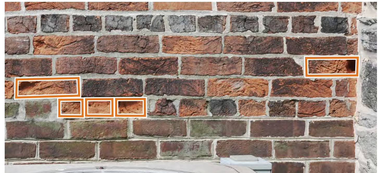
A BRICK REPAIRS REPRESENTATIVE PHOTO SHOWING EXAMPLES OF BRICK FACES IN NEED OF REPAIR. PATCH DAMAGED BRICK FACES w/ TINTED MORTAR OR APPROVED PATCHING MATERIAL. SEE ELEVATION PHOTOS FOR DOCUMENTATION OF LOCATIONS.
