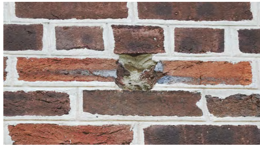
C BRICK REPAIR CLEAN OUT HOLE IN BRICK, REMOVE FILLER. PATCH BRICK FACE WITH TINTED MORTAR OR APPROVED PATCHING MATERIAL, AND RESTORE MORTAR JOINTS
