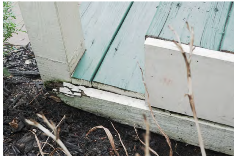
C WOOD REPAIRS DUTCHMAN REPAIR ROTTED AREA OF SKIRT BOARD AT STOOP.
